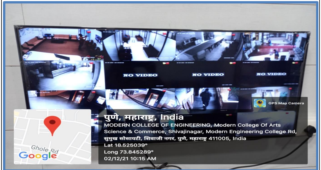
Central CCTV room
