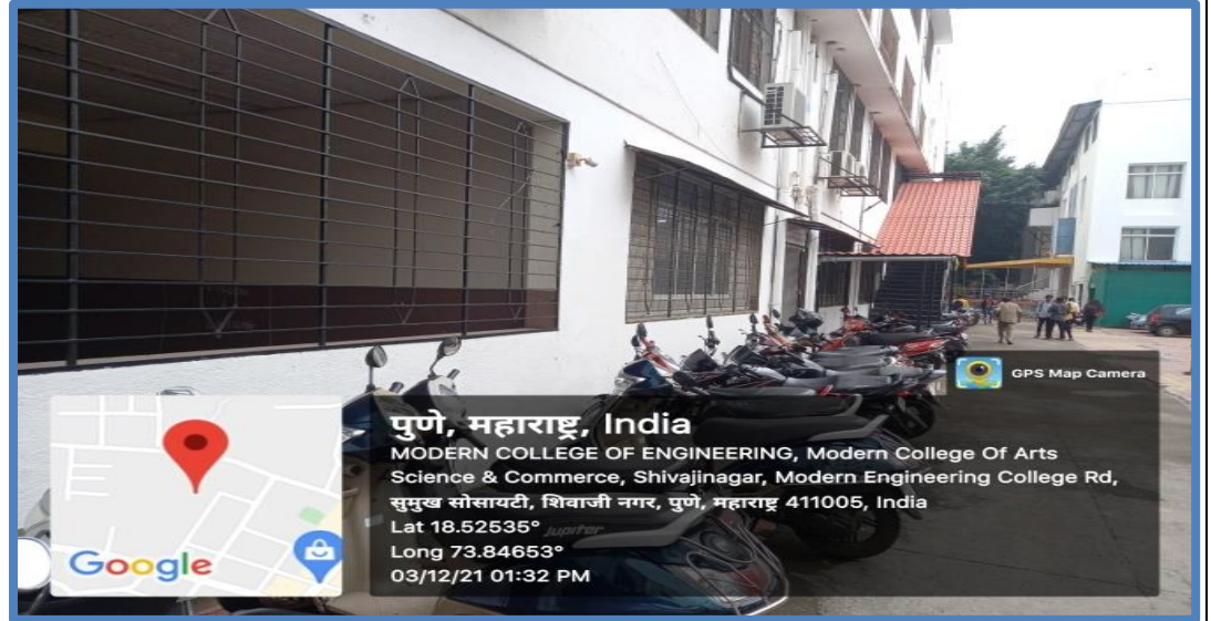
CCTV Installed at various area in campus
